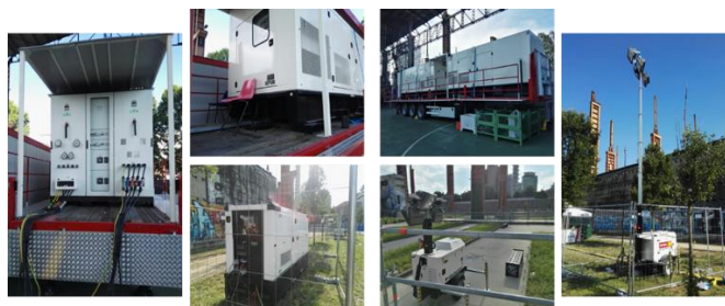
Figure 9. Gensets installation during the KappaFuturFestival (Turin_Parco Dora 6-7th July 2018).
